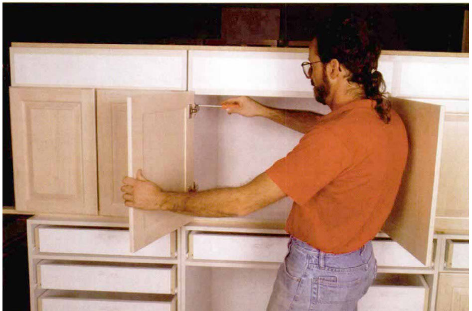
Installing the doors. Once the boxes are assembled, Fratrack snaps the doors onto their hinges and tinkers with their final positioning with a screwdriver. Sink bases make up the top tier of cabinets. They sit atop a row of base cabinets.
